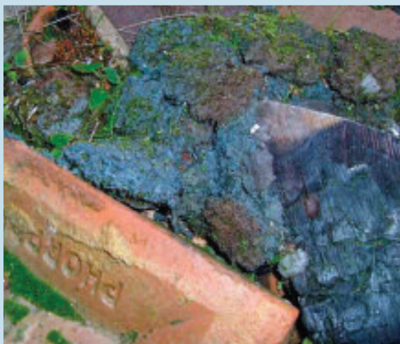
Blue asbestos in the rubble from the fire.
