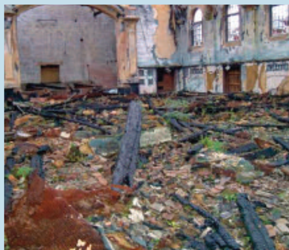
West Park Hospital after the fire and before decontamination.
